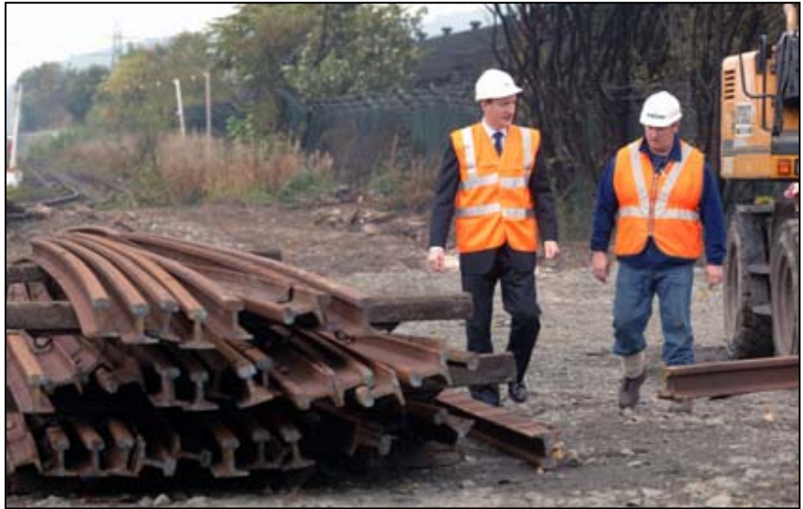
ACTION MAN: Scottish Transport Minister Tavish Scott seeing a rail reopening project under way with construction manager Andy Nisbet near Alloa
