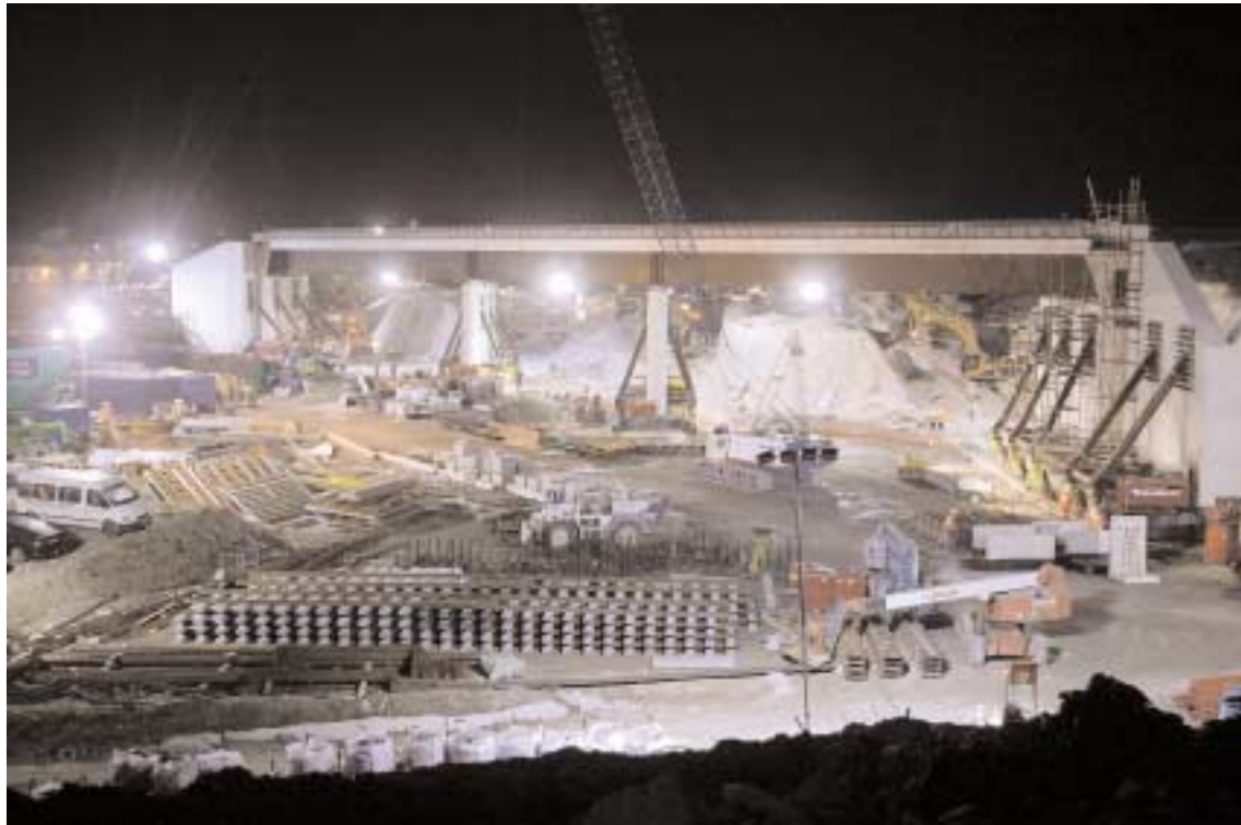
RAIL ON RAIL: Britain's first high-speed rail line is taking shape. This picture shows a 9,000 tonne new bridge being constructed in North Kent in May to take the line from Gravesend to London over the new line from Ebbsfleet to Stratford
