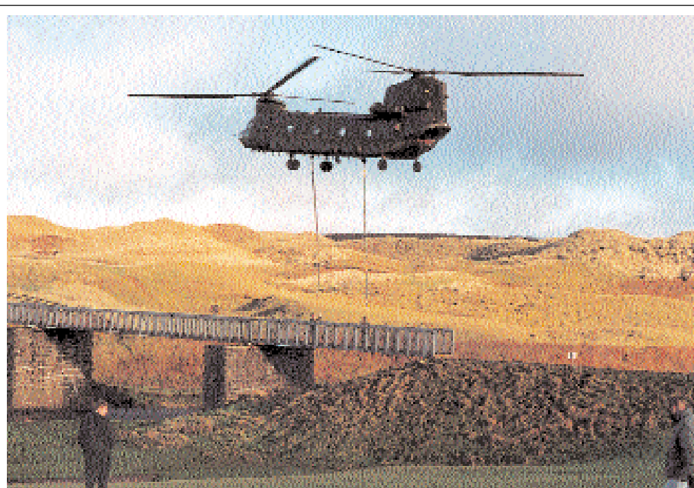
The Army and the RAF came to the rescue when a bridge needed replacing on the Giant's Causeway and Bushmills Railway being built on the route of an old tramway in Northern Ireland. This twin-rotor Chinook helicopter lifted out the existing bridge as a crowd of 200 people from the nearby village of Portballintrae watched. The new bridge goes in in April and the railway begins operations in June. Visitors should head for Coleraine (by bus or train from Belfast) where an open-top bus will take them to the railway. The holiday resorts of Port Rush and Ballycastle are nearby. Details: 012657 41157
