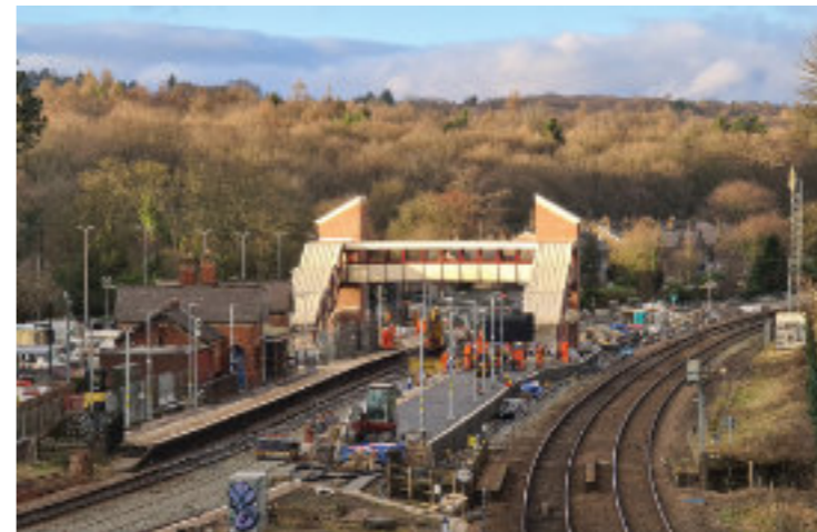
ACCESSIBLE FUTURE: Lifts are installed at Dore & Topley station
