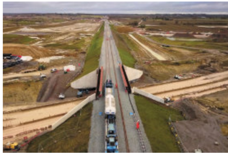
CALVERT: One of the most significant locations for Britain's railways in 2024. Two new railways are being created in Buckinghamshire. The recently completed bridge will carry East West Rail over High Speed 2's London-Birmingham Picture: East West Rail
