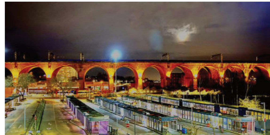
Network Rail is seeking planning permission to repair the 27-span Stockport viaduct over the river Mersey because some of its estimated 11 million bricks are crumbling and other safety measures are needed. Nearby, work is continuing on a new transport interchange to replace the old bus station and to create "improved links to the rail station". The interchange is scheduled to open in March
