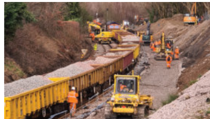
BIG DIG: The cutting near Dore is widened for an extra track
