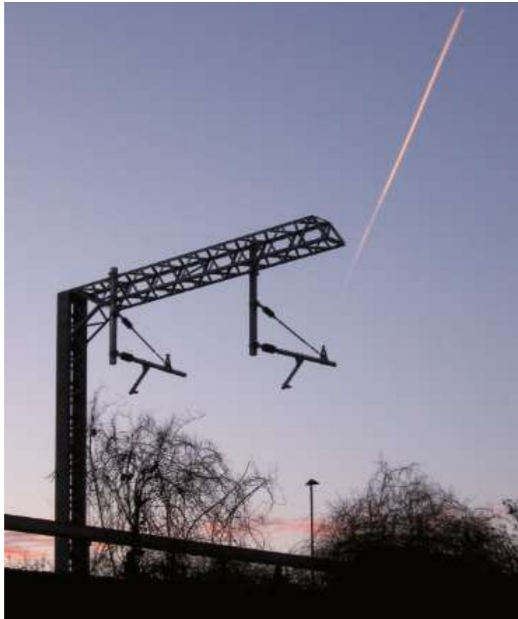
WAITING FOR WIRES: The Carmarthen service will use bimode trains as electrification goes only as far as Cardiff on the main line from London. This gantry is on the Cardiff City line, part of the South Wales metro
