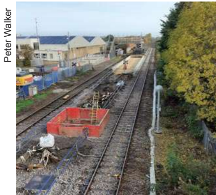
BILLINGHAM: Looking north along the Coast route towards Newcastle. The orange square between the tracks is probably for one of the lift shafts
