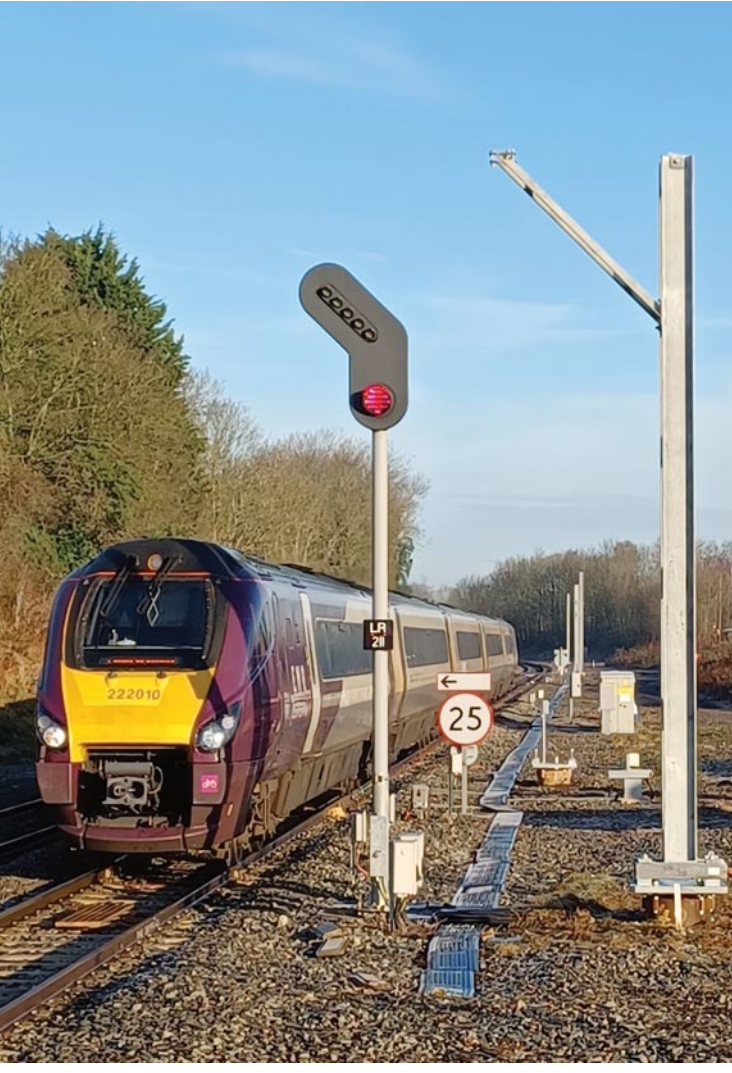
A diesel passenger train nearing the platform at Market Harborough station, past recently installed electrification masts
