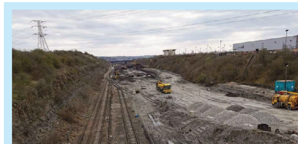
SHEFFIELD: A new future is carved out of the former Tinsley marshalling yard
