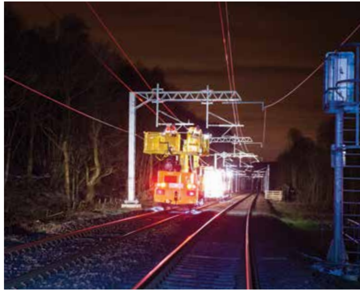
SCOTLAND SHOWS THE WAY: Work to electrify the Glasgow-Edinburgh line via Falkirk Grahamston. There will soon be five electrified routes between the two cities. Manchester, Leeds and Sheffield will have to make do with diesels – and dreams
