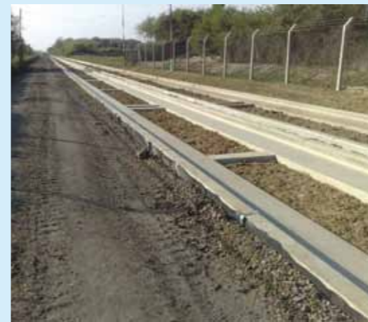
WASTED ASSET: The guided busway under construction in 2009 on the trackbed of the Cambridge-St Ives line
