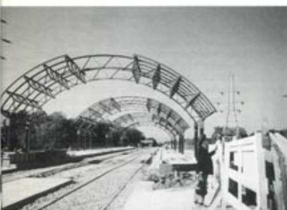
Station for the Dallas suburb of South Oak Cliff is built. By 1997 the light rail system will be operating
