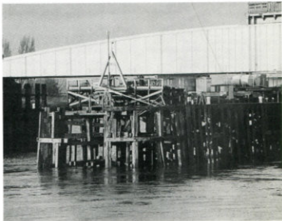
The much battered bridge at Goole.
