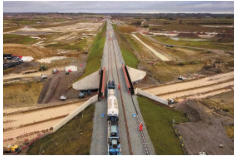
CALVERT: One of the most significant locations for Britain's railways in 2024. Two new railways are being created in Buckinghamshire. The recently completed bridge will carry East West Rail over High Speed 2's Picture: East West Rail
