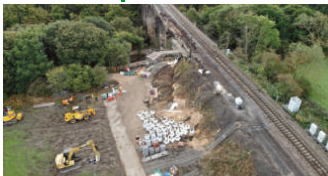
The damaged Plessey viaduct
