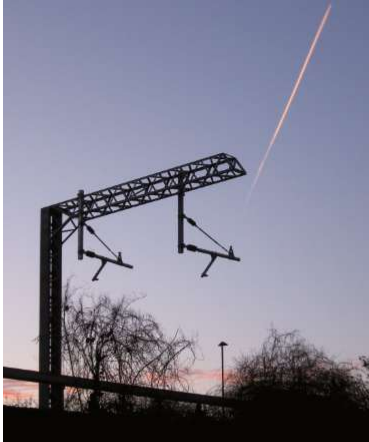
WAITING FOR WIRES: The Carmarthen service will use bimode trains as electrification goes only as far as Cardiff on the main line from London. This gantry is on the Cardiff City line, part of the South Wales metro
