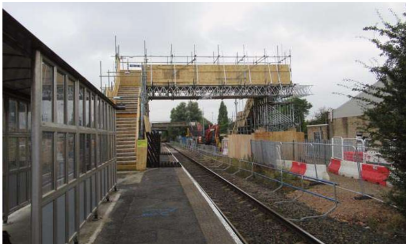
BILLINGHAM STATION: Looking south towards Stockton and Middlesbrough with one new footbridge in place.
