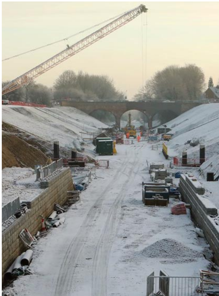
FROZEN HEART: Platforms were being constructed as snow fell in December last year at Winslow station which will be at the heart of East West Rail when it transforms travel between Oxford, Milton Keynes and, eventually, Cambridge. More than 500 pre-cast concrete platform units were lifted into position using a crane with a boom longer than Nelson's Column
