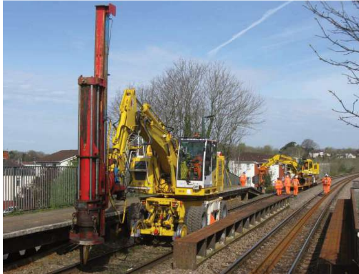
Two machines for driving piles into the ground working at Waun-Gron Park station on the Cardiff City line in April, part of the work to electrify the core valleys lines
