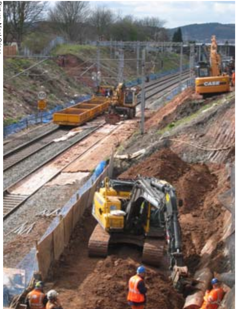
BIG DIG: Four tracks are being squeezed into this cutting west of Tamworth on the existing two-track Trent Valley line
