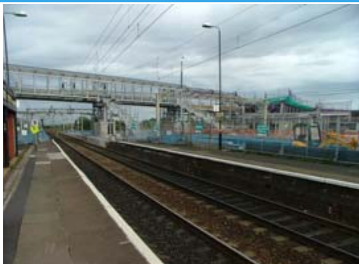
Station rebuilding and new link bridge work at Allerton station in June 2005.
