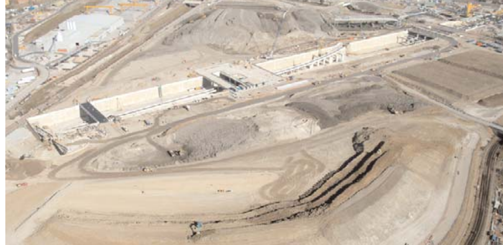
The vast engineering work under way at Stratford, east London to build the international station for the Channel Tunnel rail link. The line goes through Stratford in a tunnel.
