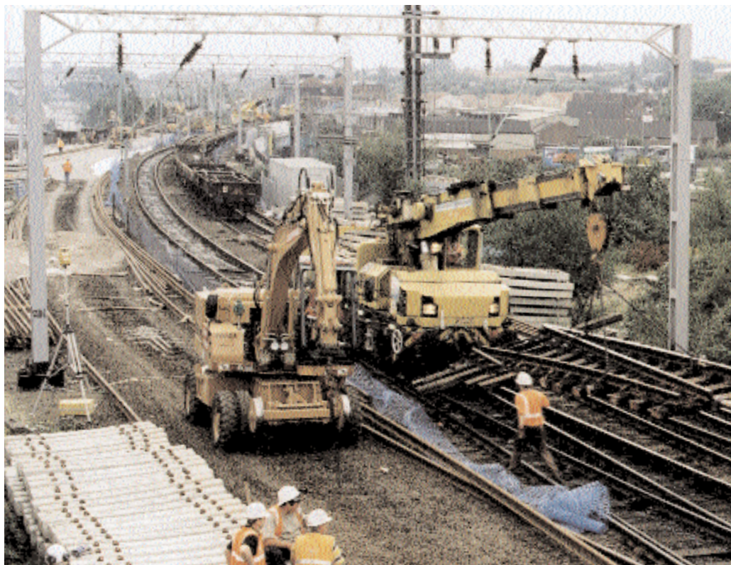
ACTION: Railtrack's core responsibility was to maintain and improve the track and infrastructure. Some projects like this one at Proof House Junction, Birmingham, did happen. Many more were delayed or shelved.
