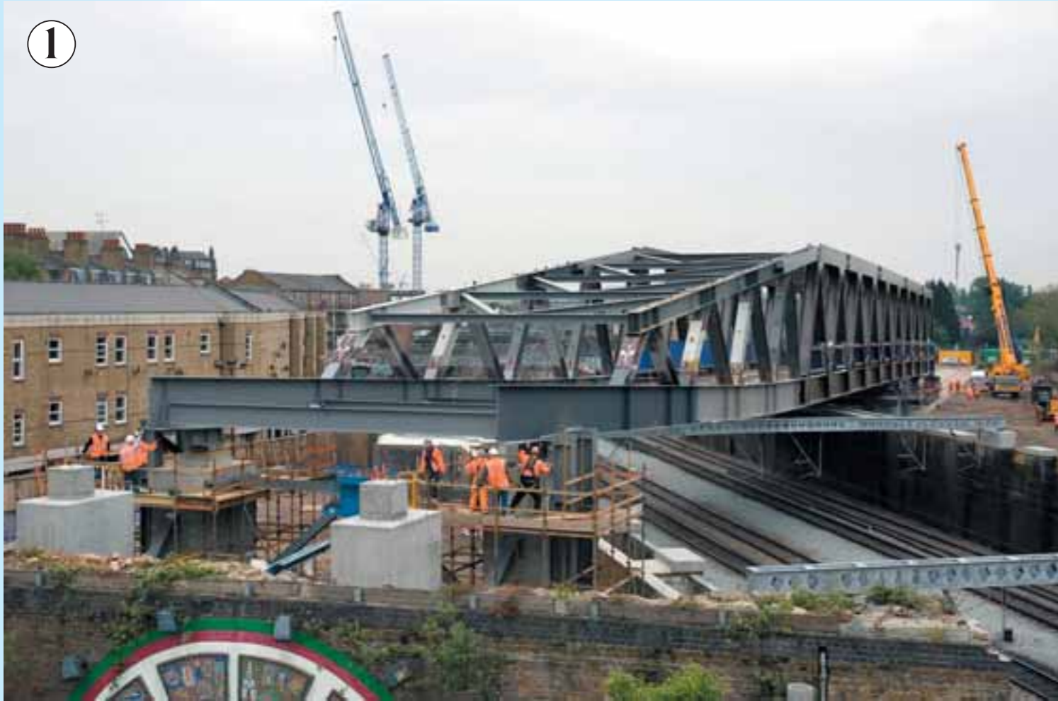
BRICK LANE: The Great Eastern main line came to a halt over the bank holiday weekend of 4 May while this 800-tonne bridge was shunted into place. A few weeks later the main line was closed again when scaffolding or concrete reportedly fell on to the tracks
