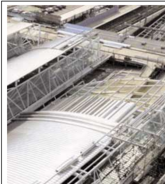
The roof of Leeds station is being renewed as part of the Leeds First scheme. Railtrack says the station will be lighter, brighter and better ventilated as a result. Rail travellers will be relieved when the work is completed having suffered delays and problems for over two years.
